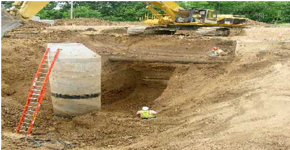
Figure 4.4: Excavation work can be incredibly hazardous (OSHA)
