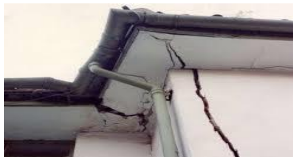
Figure 1.2: Expansive soils in building deterioration (Sitar, 2012)
