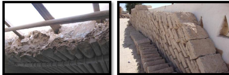
Figure 3.7: The ceiling with stumps of palm trees, and small stones. The Bricks are made with clay materials which are dried in the sun, this ceiling has a dimensions of 40 x 30x 10 cm (Shahran, 2018)
