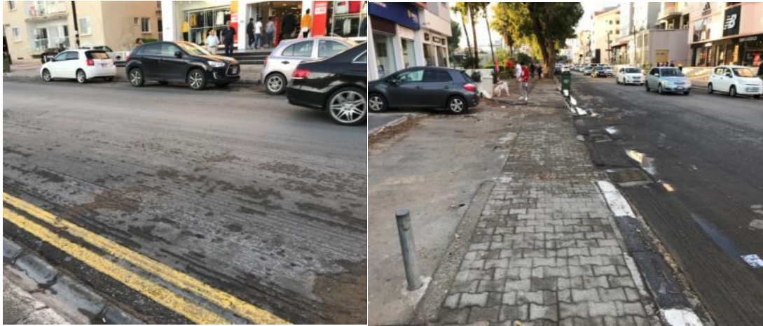
Figure 4.8: Road condition in Ismet Inonu Boulevard
