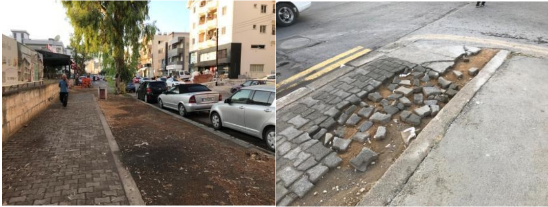
Figure 4.5: The condition of sidewalks in Ismet Inonu Boulevard
