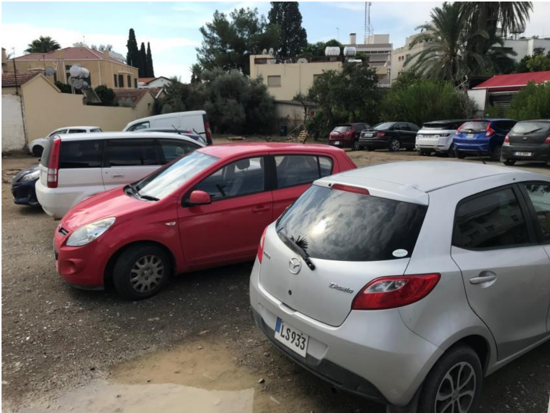
Figure 4.19: A poor conditioned parking lot space in Osman Pasa Street
