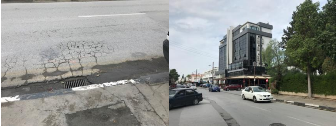
Figure 4.18: Road condition in Osman Pasa Street
