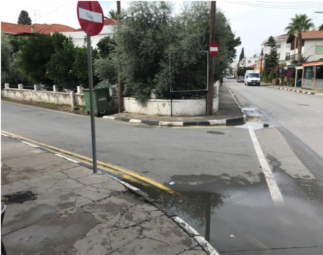
Figure 4.17: A disconnected sidewalk segment in Osman Pasa Street
