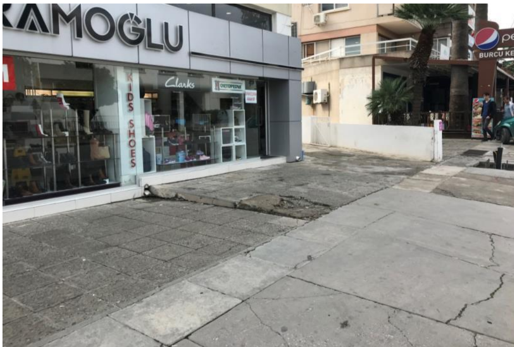
Figure 4.14: Sidewalk Condition in Osman Pasa Street
