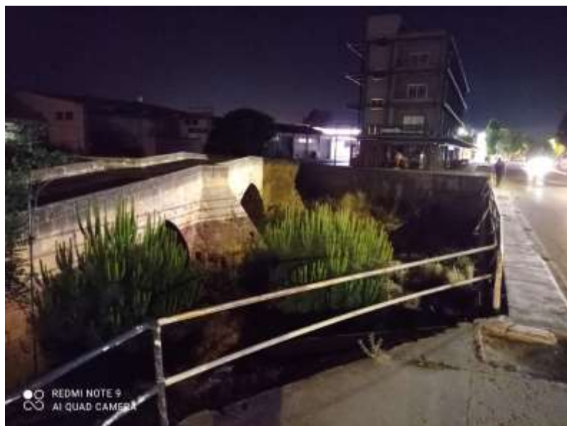
Figure 5. 15: Old Bridge for crossing the river and the new urban one which looks risk to the residents, Main Tributary, Galibolu area –Lefkosa –Nicosia
