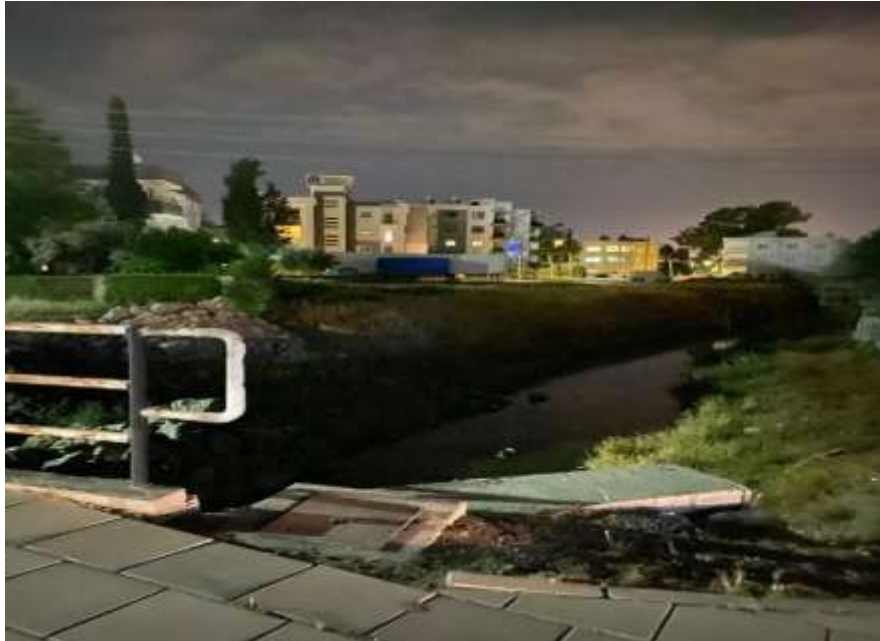
Figure 5. 13: A broken structure, and isolation of the river with a cracked dangerous pavement, Tributary one, Marmara area, –Lefkosa –Nicosia
