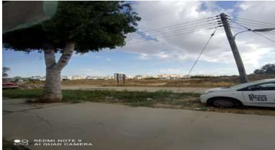
Figure 5. 14: An extraction work for a the soil is ongoing within the river edges, Tributary two Ortakoy area –Lefkosa –Nicosia
