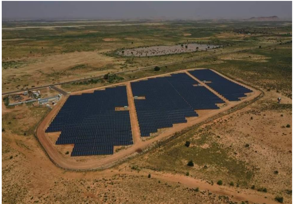
Al Fashir 5 MW Solar PV Power Plant
