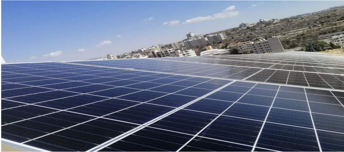
Figure 3. 7: Photo Voltic panels for solar energy generation on the roof of AMQF building (Photo: L, Arafa, 2021)
