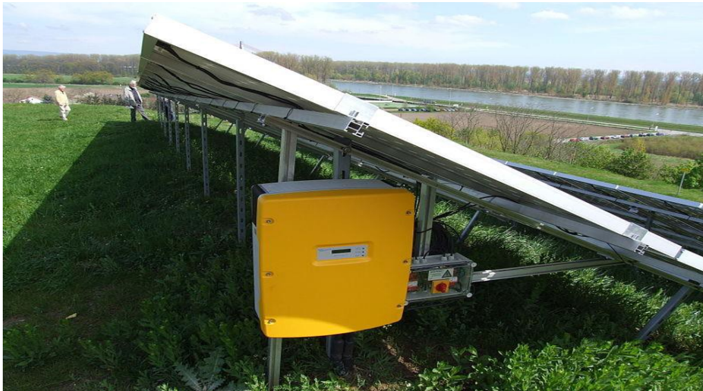
(Figure 4.6: An inverter for solar mounted free standing planet alongside with Rhine )
